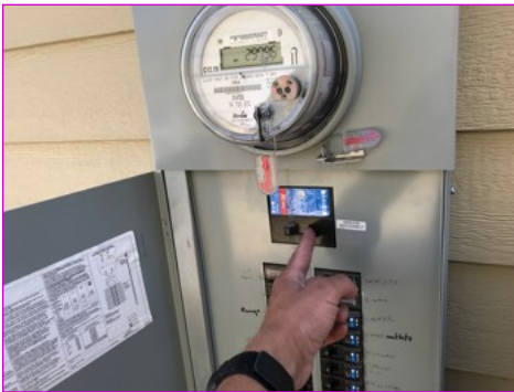
SERVICE PANEL Main Disconnect
