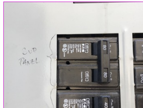
80 AMPs at sub panel
