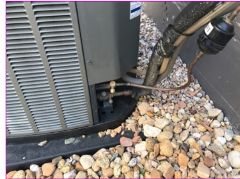
CENTRAL AIR CONDITIONER AC Refrigerant Lines
