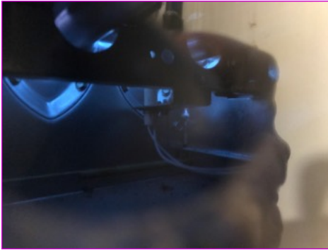
FURNACE Combustion Chamber
