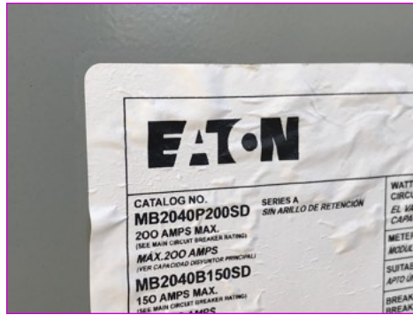
SERVICE PANEL Service Panel Manufacturer
