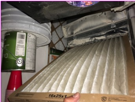
FURNACE Furnace Air Filter
