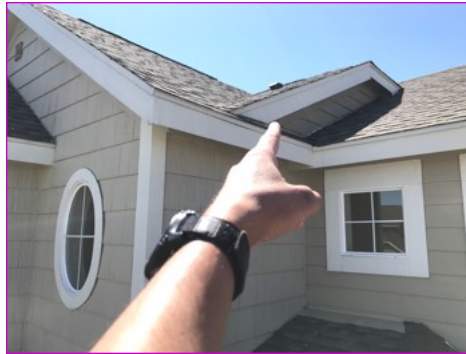
Inspector suggests sealing with sealant or foam at the soffits on the upper right side of the roof to prevent pest intrusion to the attic space. Gap present at flashing.
