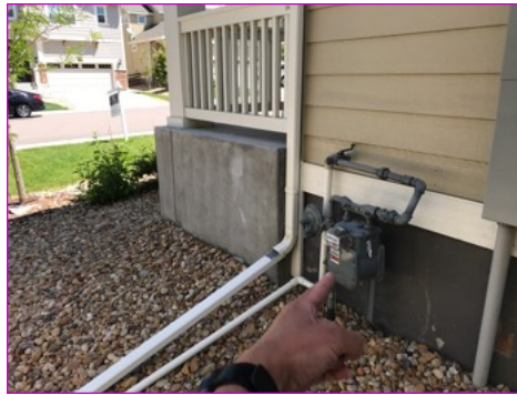
GAS SYSTEM Gas Meter
