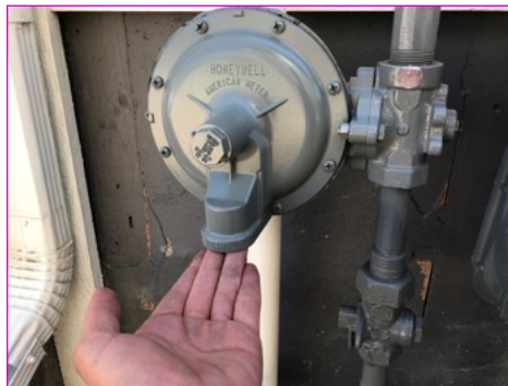
GAS SYSTEM Gas Regulator
