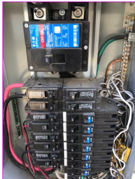
SERVICE PANEL Cabinet Condition
