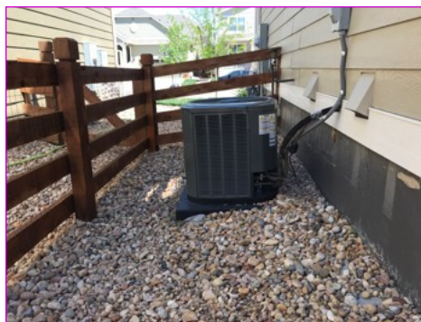
CENTRAL AIR CONDITIONER Compressor Unit
