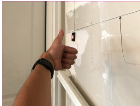
OVERHEAD GARAGE DOOR Automatic Opener Switch
