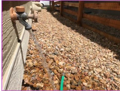
EXTERIOR PLUMBING Exterior Faucets
