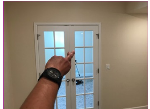
French door in the basement is tight and rubs together. Suggest correction/shaving or sanding the door.
