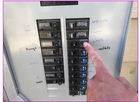
The breaker to the washer did not function properly when tested at the button at the outside service panel. The inspector suggests replacing this a AFCI/GFCI breaker by a professional electrical contractor for safety.
