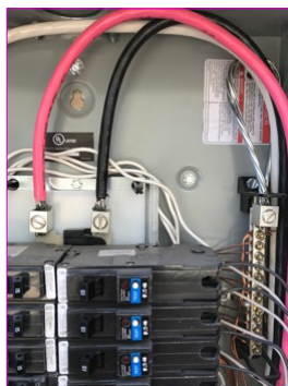
SUB-PANEL Feeder Conductor Condition
