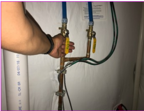
WATER SUPPLY PIPES Main Water Shut-off
