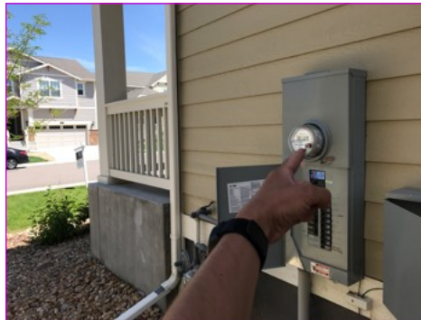
ELECTRICAL SERVICE Electric Meter Location
