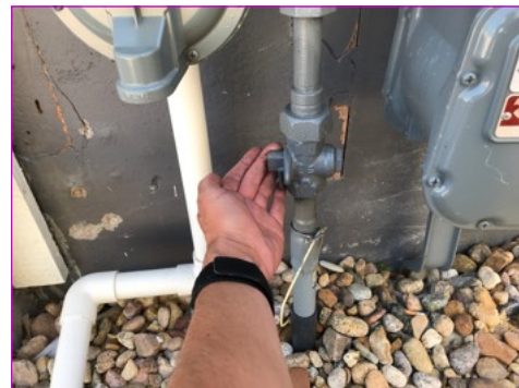
GAS SYSTEM Main Gas Shut-off
