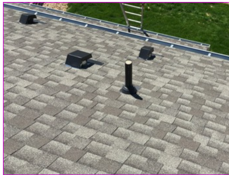
SYSTEM VENTS Plumbing Vents
