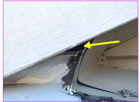
Inspector suggests sealing with sealant or foam at the soffits on the upper right side of the roof to prevent pest intrusion to the attic space. Gap present at flashing.
