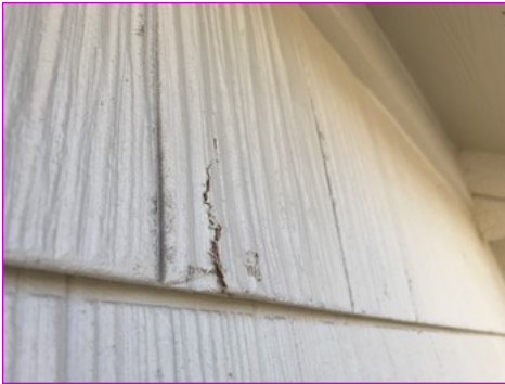
Seal and minor touch-up needed at the exterior.
