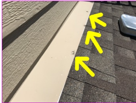
Be sure to maintain the sealant over the exposed nails at the flashing about the rear patio.
