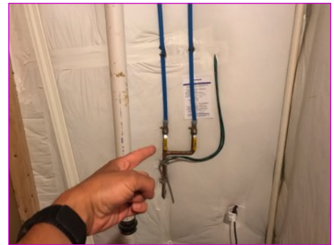
WATER SUPPLY PIPES Main Water Shut-off
