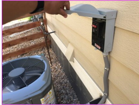
CENTRAL AIR CONDITIONER AC Electrical Disconnect
