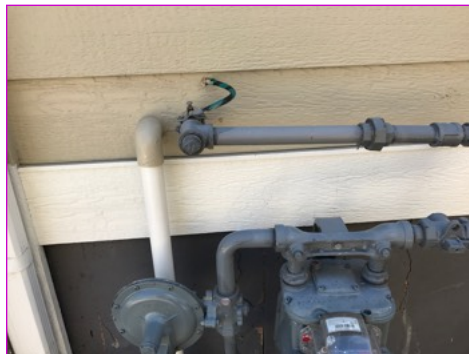
GAS SYSTEM Gas Pipe Bonding
