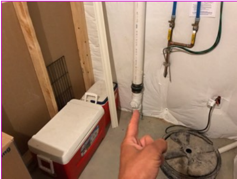
DRAIN, WASTE, and VENT PIPES Cleanouts
