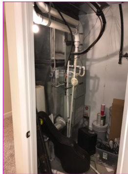
FURNACE Furnace Location
