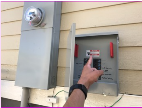
SUB-PANEL Sub-panel Location
