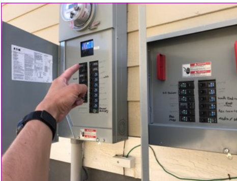
SUB-PANEL Panel Disconnect
