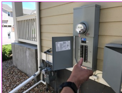
SERVICE PANEL Service Panel Location
