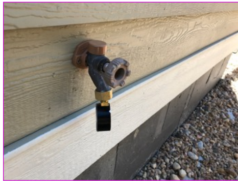
EXTERIOR PLUMBING Water Pressure
