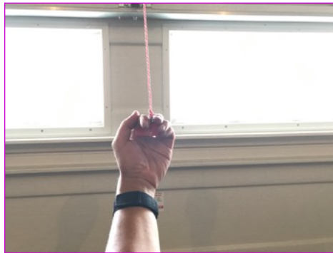
OVERHEAD GARAGE DOOR Manual Disconnect
